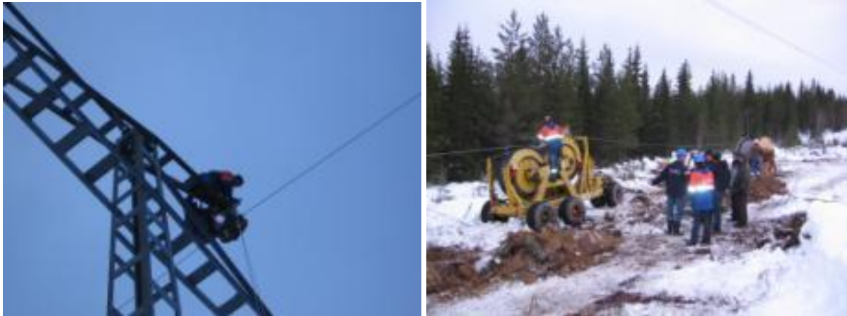
Figure 4 Laying out the ground wire on the pulley blocks (left) and work place with puller and cable drum battery – works executed in Sweden (picture by B.Dudek)
